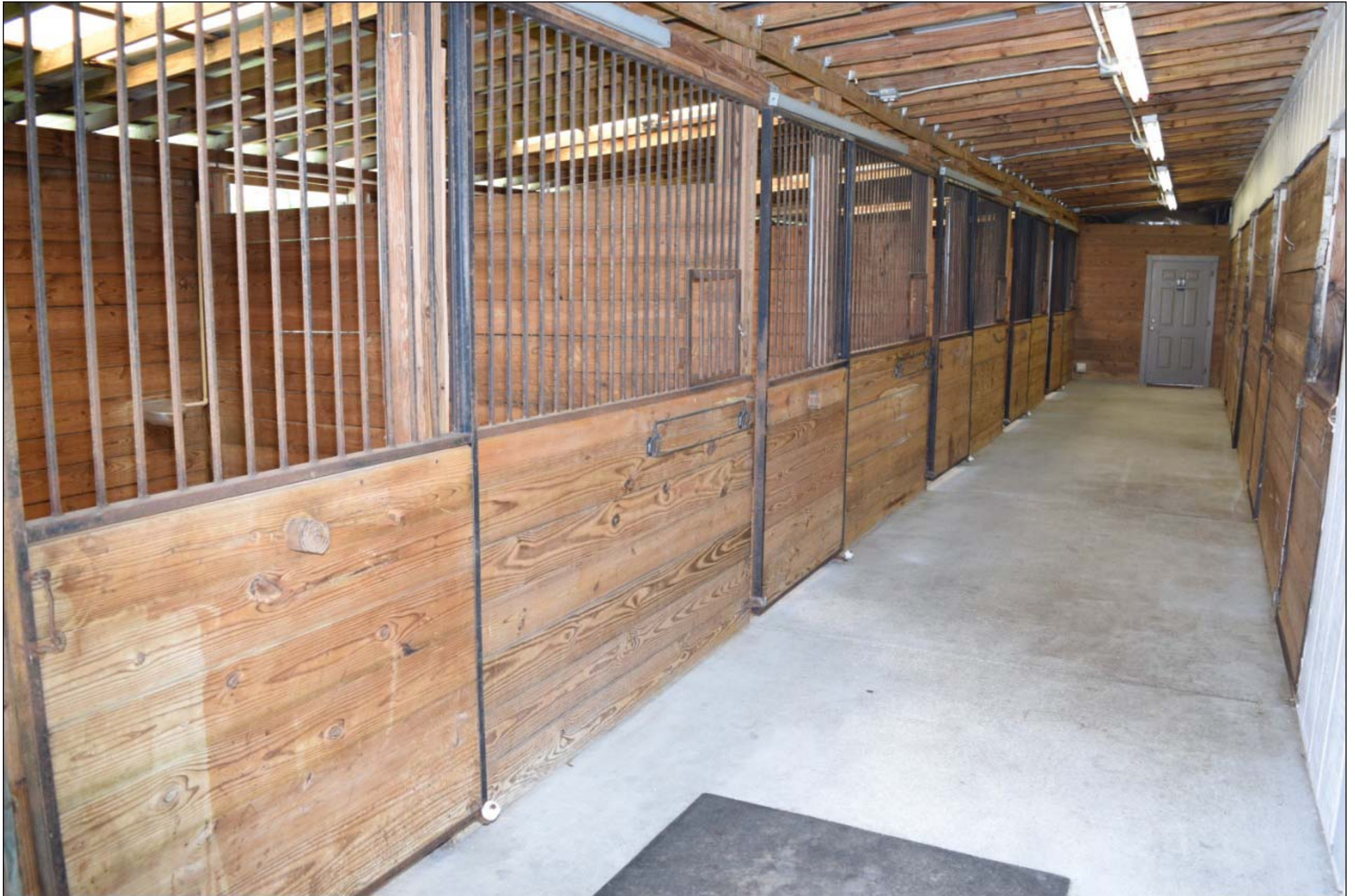
Barn West wing with ' back external windows ' – East wing is the same
